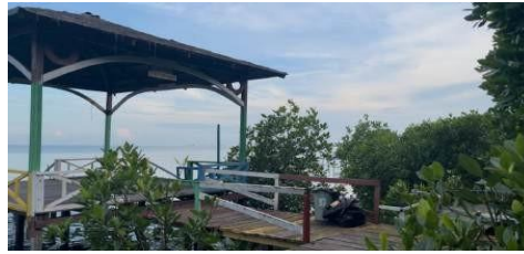
Figure 6. Actual condition of gazebos and trash cans
