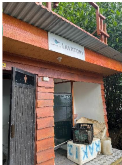
Figure 5. Actual condition of toilets
