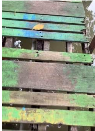
Figure 4: Actual condition of the Bridge Path: Some damage has occurred
